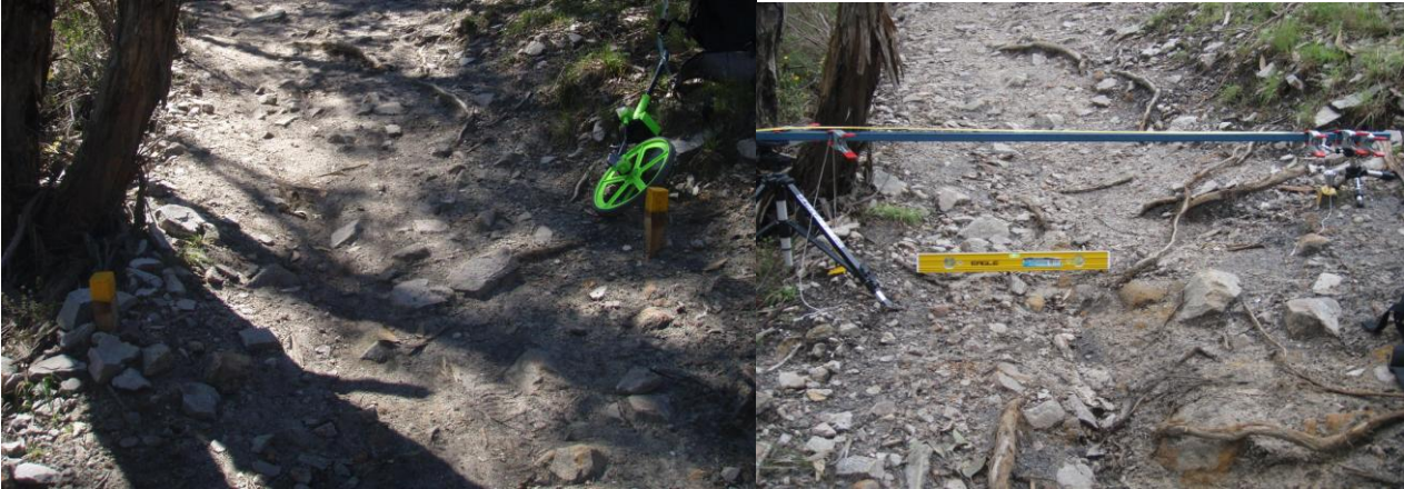
Figure 16 TV-10 in September 2008 and September 2009 showing the effects of soil movement
